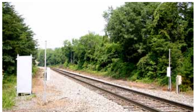
Lineside detectors serve many functions. In plastic boxes along each side of the track, these car-tracking detectors are on the Norfolk Southern line near Manassas, Va.
