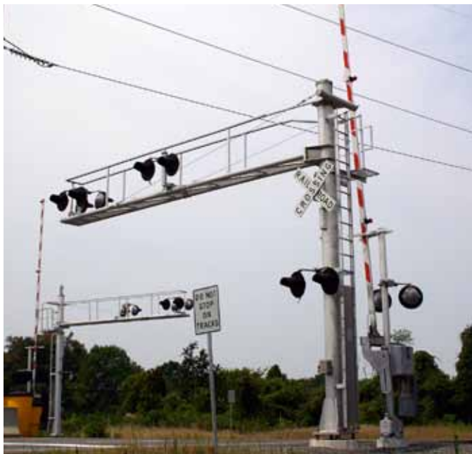
Modern grade crossings, such as this one in Manassas, Va., feature crossbucks and crossing gates. Many railroads now place flashing signals in cantilevered bridges.
