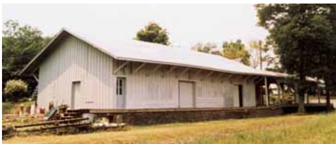
The old PRR right-of-way is still visible in front of the freight house. Note the inclined freight platform.
