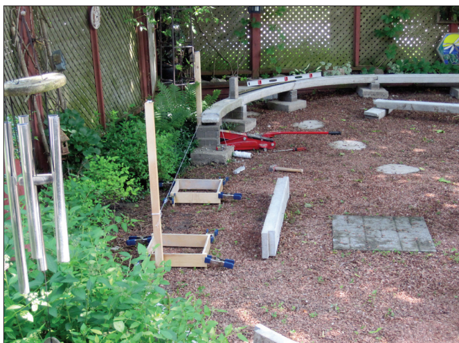
10. Footing forms in the foreground are held together with spring clamps, ready for the pour. A string is in place where the roadbed will go. A straight span is on its side at the right.
