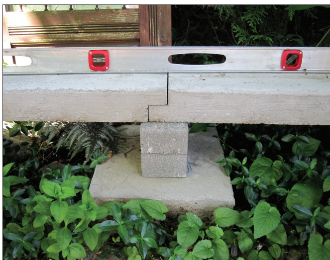
12. Spans rest on the risers without actually being attached.
