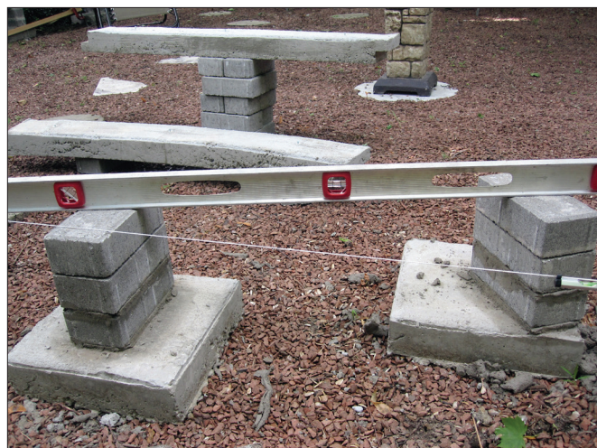
11. A mason's line is used to guide the placement of the risers. Mortar is used to bring the risers to their proper height. A line level can be seen at the far right of the picture.
