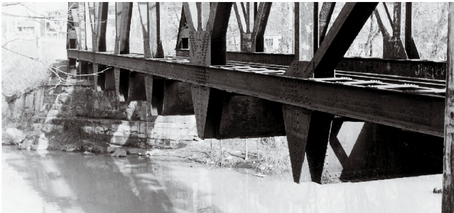
Fig. 5 Cross girder. All truss bridge designs are just different ways of supporting the cross girders under the track. This Susquehanna through truss bridge has floor beams fastened below the bottom chord at the end of each panel. The stringers that support the ties are riveted to the floor beams.
