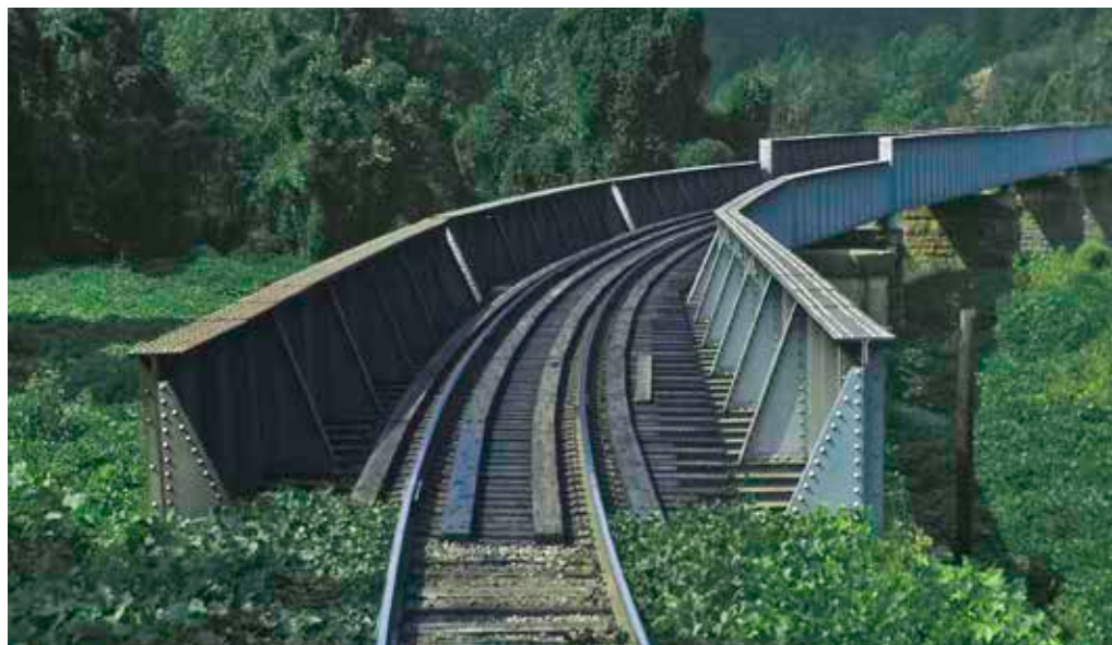
Fig. 3 Through-girder bridge. A through girder bridge is a plate girder with the beams moved up and out to provide more clearance underneath. This curved Clinchfield (CSX) bridge is made from a series of short straight bridges.
