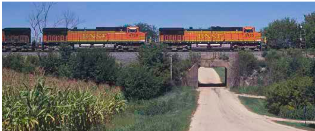
Fig. 7 Concrete viaduct. Box-style concrete viaducts, like this example in Illinois, are an inexpensive way to span a small road or stream. Carl Swanson photo
