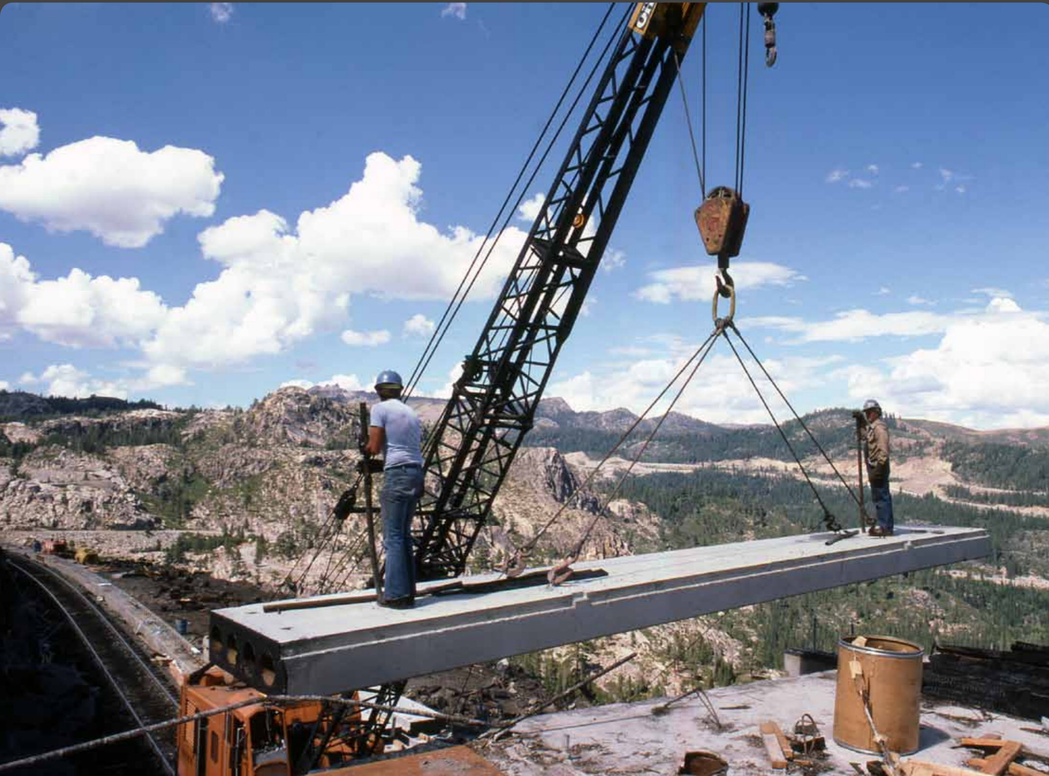
The first roof panel for concrete snowshed 37 goes on. The two laborers pictured will line up the roof slab holes with vertical threaded rods and then bolt the panel down.
