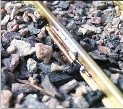
Soldered rail joints offer the most reliable electrical connection.
