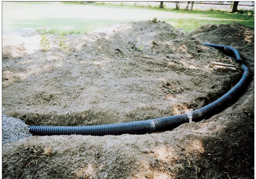
Due to the amount of moisture present in upstate New York, I used 4" perforated drain pipe beneath the track to carry away excess water and cut down on frost heave issues.
