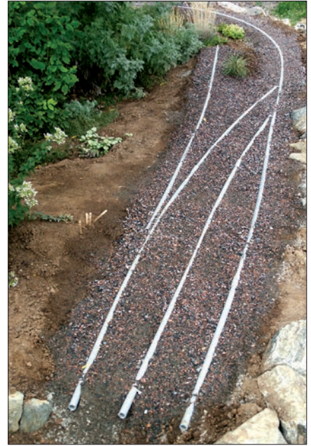
Once the trench is filled with gravel and tamped, it's ready to have the track attached.
