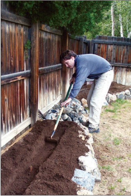
A regular garden hoe works well for trenching out the subroadbed. Allison Strong
