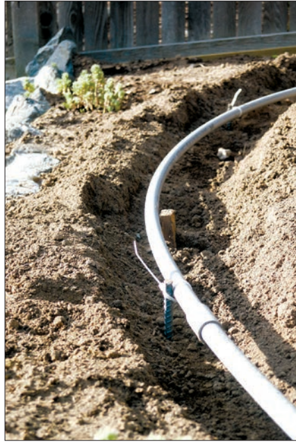
I used PVC electrical conduit set in a trench as an anchor for the track on my Tuscarora Railroad.
