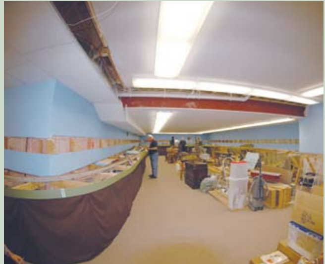
Jeff Otto extended the basement under a four-car garage to create a generous L-shaped area for his HO scale Missabe Northern RR. A peninsula will occupy the center, and the break in the backdrop will accommodate the second level's supporting joists. Pat Student photo
