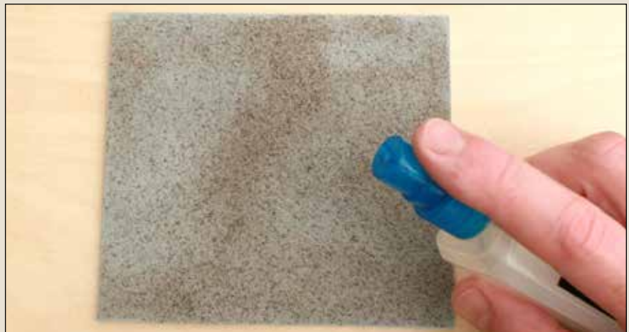
To avoid displacing the small stones, Lance uses a fine mist bottle sprayer to apply diluted matte medium to bond the ballast to the rooftop.
