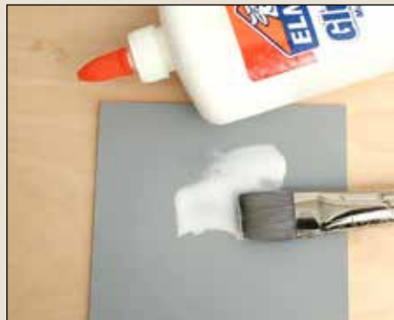
Lance first uses a 1"-wide brush to spread a thin layer of ordinary white glue over the entire rooftop surface.
