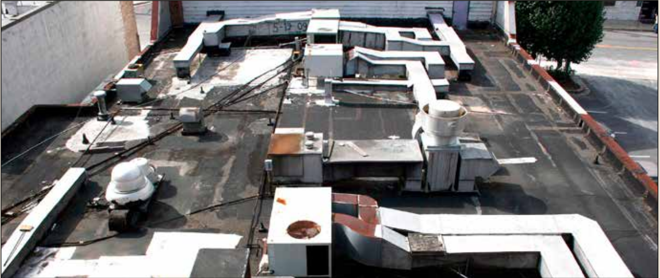
The black color and seam pattern suggest that tar paper rolls cover the roof.
