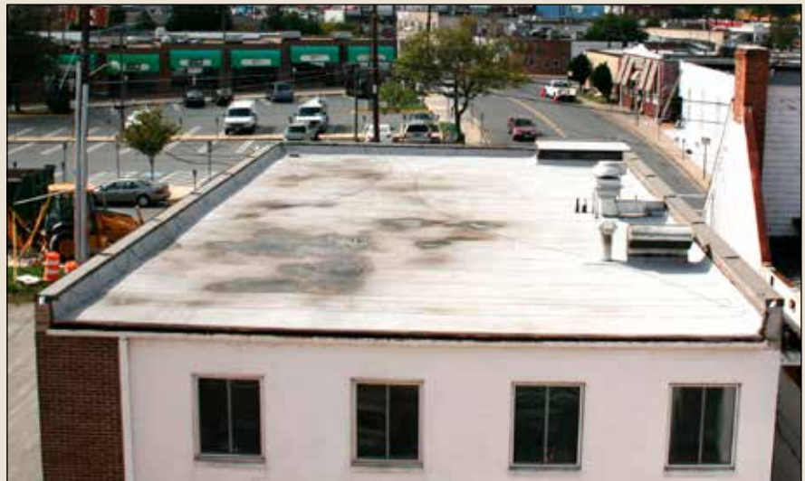
Judging by the gray color, this is probably a single-ply membrane roof surface.
