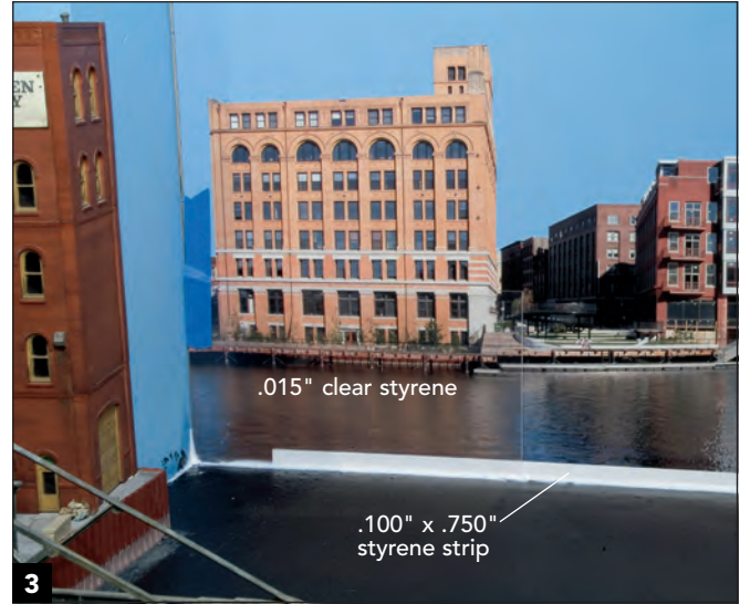
3 To contain the resin, I installed styrene dams and caulked along the seam at the bottom of the harbor. I added clear styrene to protect the photo backdrop.
