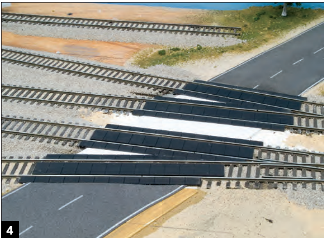
4 I installed BLMA rubber grade crossing strips, which are easy to cut and fit the irregular track angles found in the crossing.
