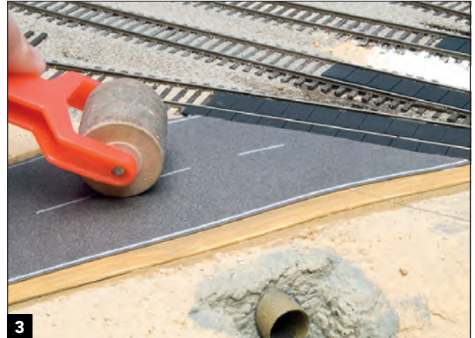
3 After the road has been positioned, use a wallpaper roller to smooth out irregularities and help ensure even adhesion of the road material to the styrene.
